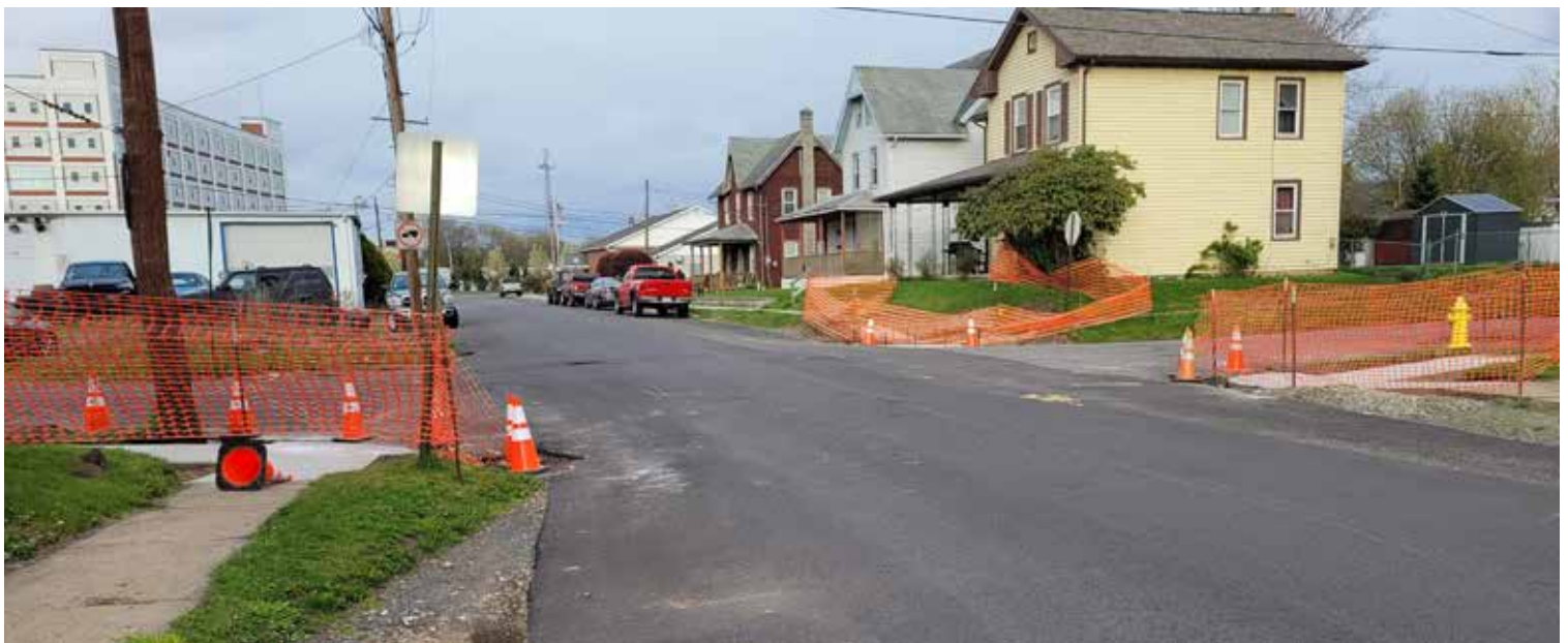
Williamsport Streets Department upgraded some sidewalks in Newberry this summer to add ramps. This is the corner of Boyd and Depot Streets.
