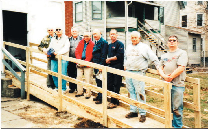
Newberry Lions All Stars (L-R) Moe Johnston, Carl Floyd, Jack Colman, Gary Klees, Ron Savits, Dion Coleman, Marc Tupper & Jim Fry went to bat for Newberry neighbor Joan Grove and built an accessibility ramp at her Cummings Street home.
