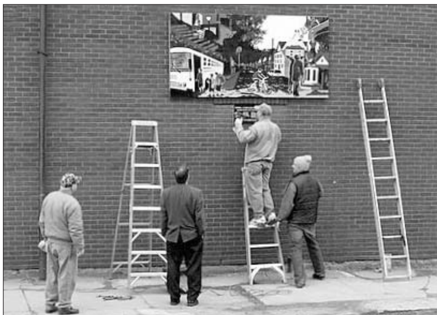
Highlighting the event was the public dedication of the mural "A Look at Our Corner of the City". Seen installing the mural is handy Chris Haberstroh , on the ladder, assisted by Bill Kieser, Jr. , and interested neighbors serving as sidewalk superintendents.
